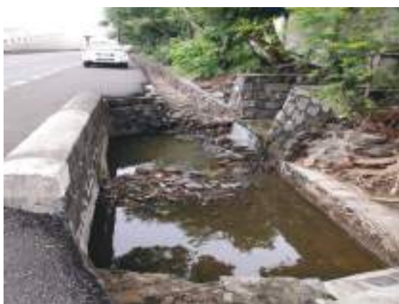
Figure 17: Road Conditions and Water Discharge before Works
