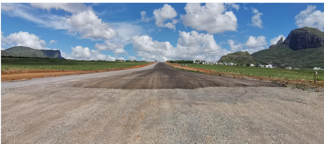
Plate 7: Laying of Base Course asphalt from Node T to Node J completed
