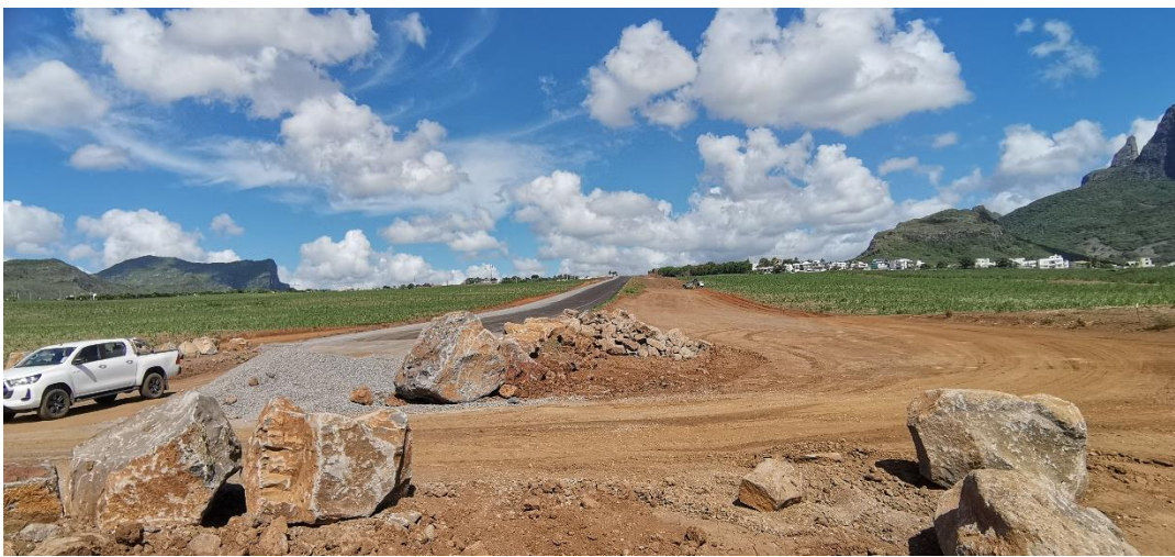
Plate 6: Laying of Base Course asphalt from Node T to Node J completed
