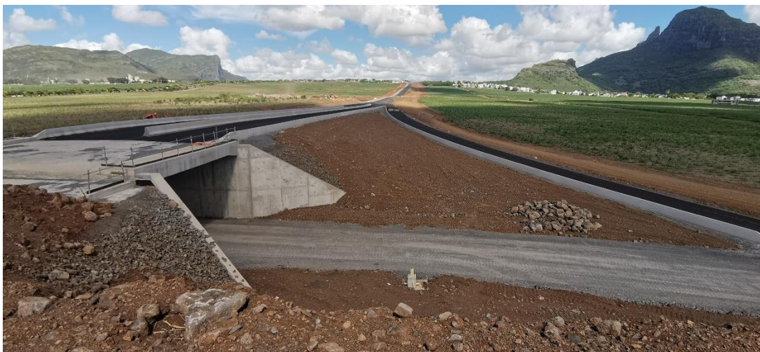
Plate 4: Ramps completed at proposed grade separated junction at Cascavelle. Prime coat laid
