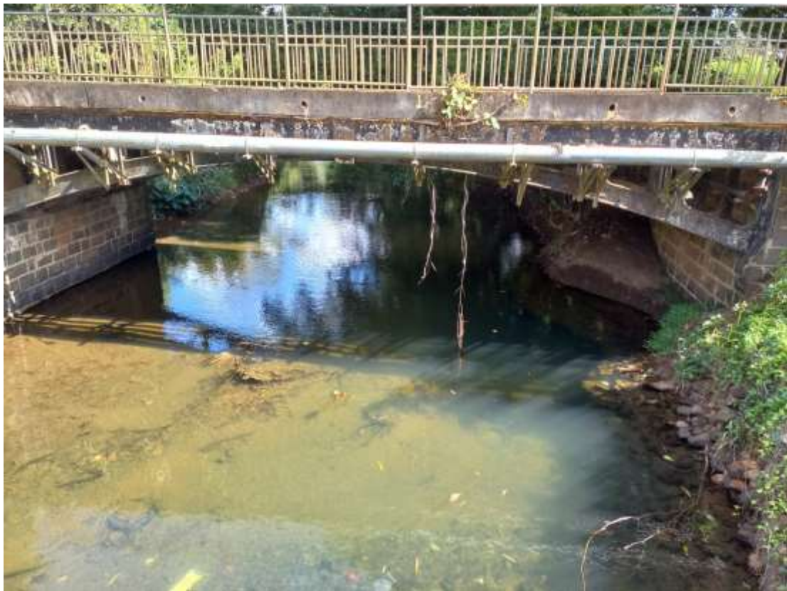
Fig 3: Sign of deterioration of steel structure of existing bridge deck
